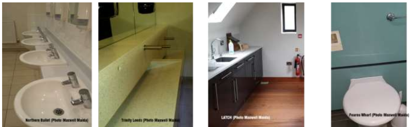
Figure 13. Water saving installations
